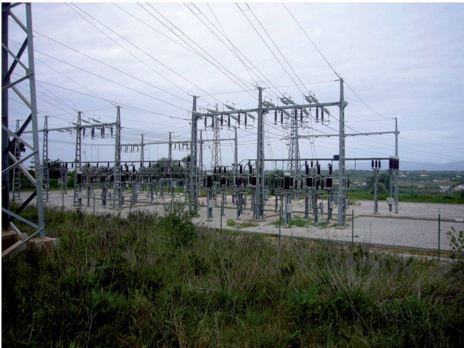
Figure 16: Substation in terrain previously used for agriculture, Algarve, Portugal (source: F. Jorge, 2013).
