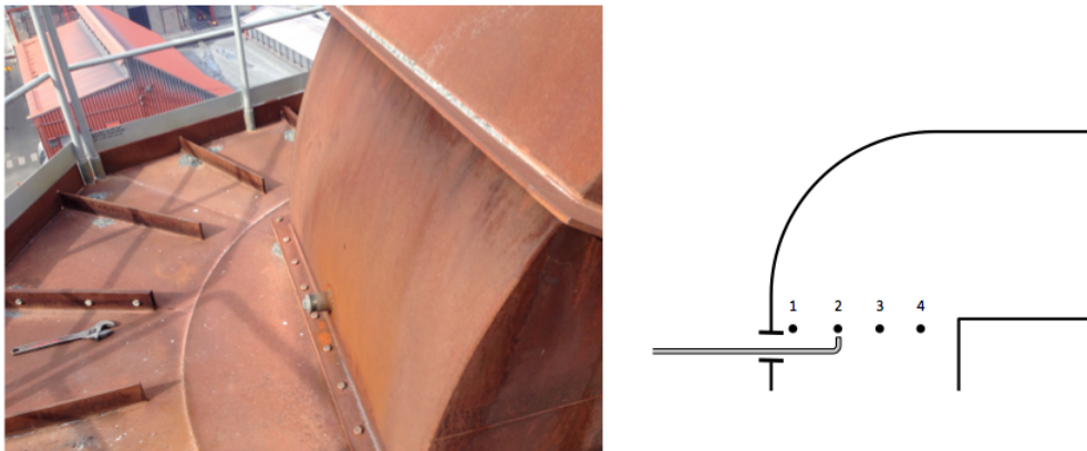
Figure 6.8: Location for taking pitot samples at the overhead duct
