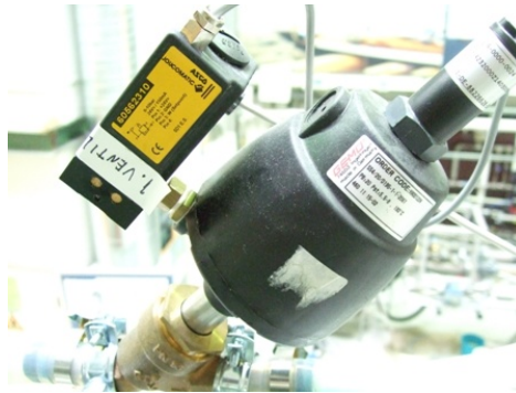
Figure 3.13: The choke valve used before the separator
