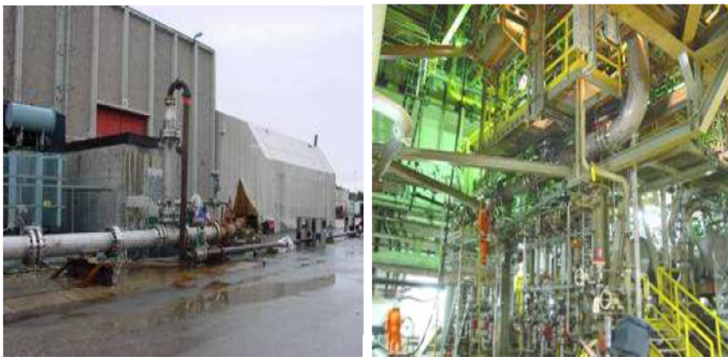
Figure 2.6: Degasser installed at the test site and off-shore on Statfjord-B platform Adapted from (Schook et al., 2005)
