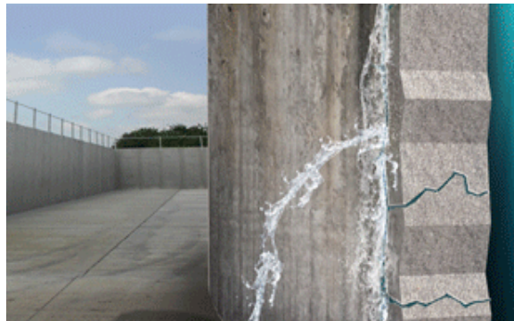
Figure 5.1: Cracking of concrete panel in a liquid-retaining concrete tank followed by a leakage, AlchemyPolymers (2015).
