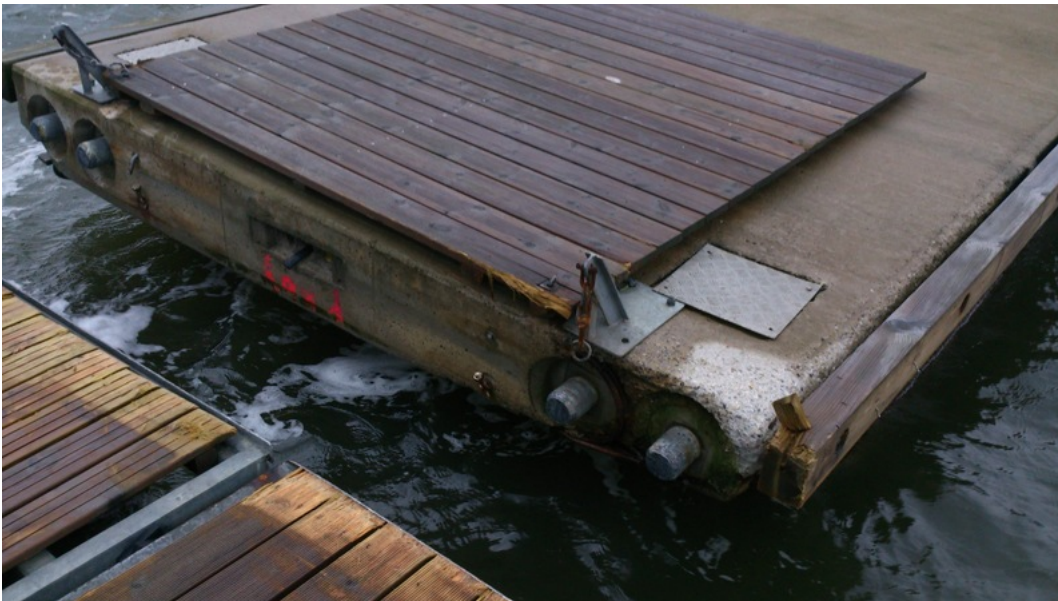
Figure 3.3: Floating dock element end. PHOTO: Bi-Brygga AS
