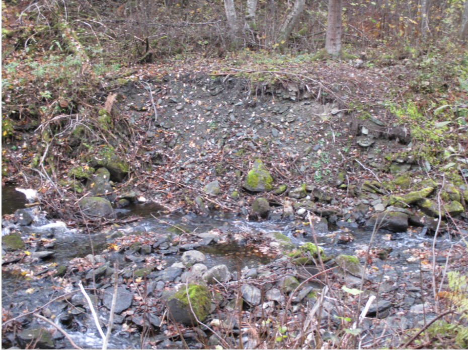
Figure 16: Observation of erosion at cross section 12
