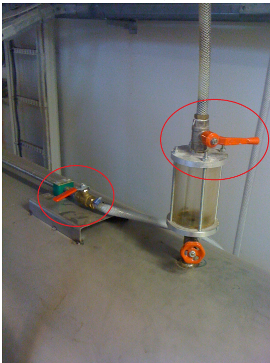
(b) Bleed valves by stairs.
