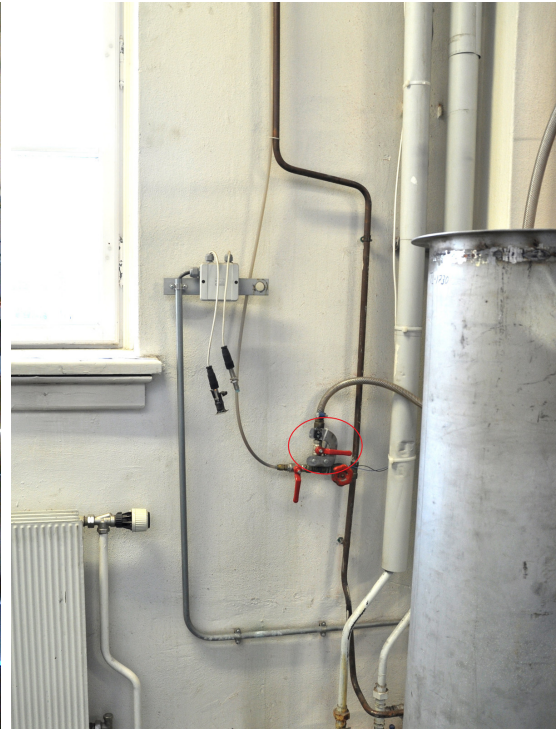
(b) Valve for vacuum pump priming water.
