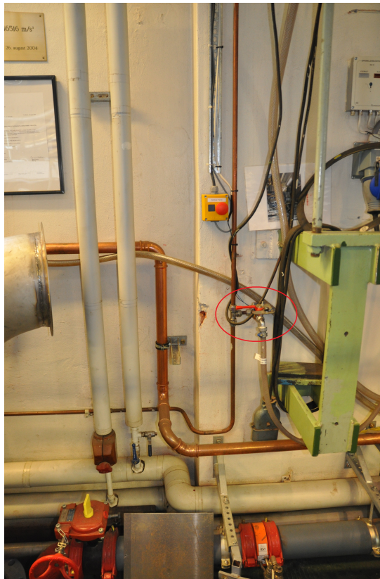
(b) Valve for cooling water for hydraulics
