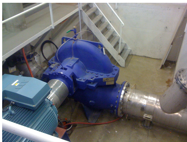
Figure 4.13: One of the feed pumps in the Waterpower Laboratory.
