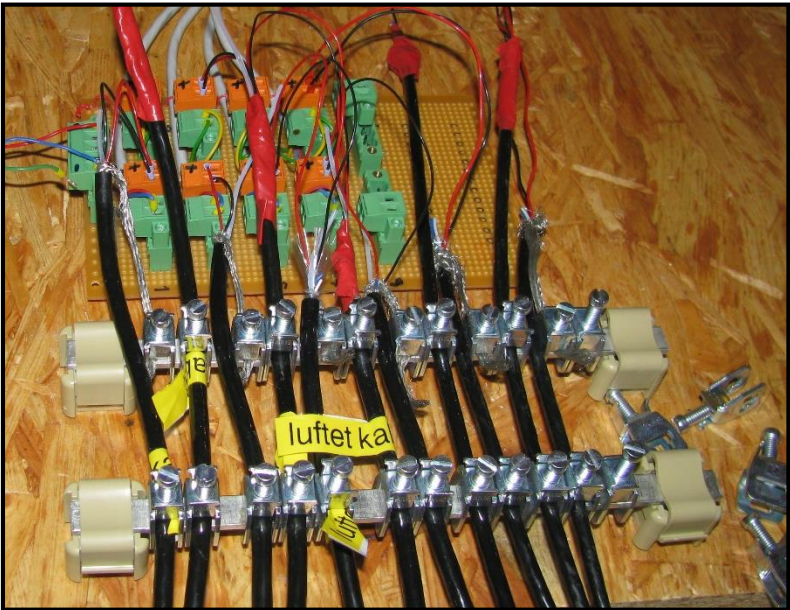
Figure 68: Chipboard for cable connection
