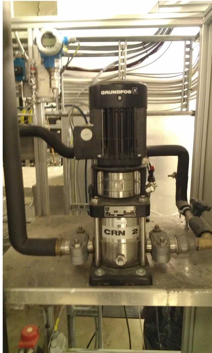
Figure 6 A GRUNDFOS pump in the expander loop
