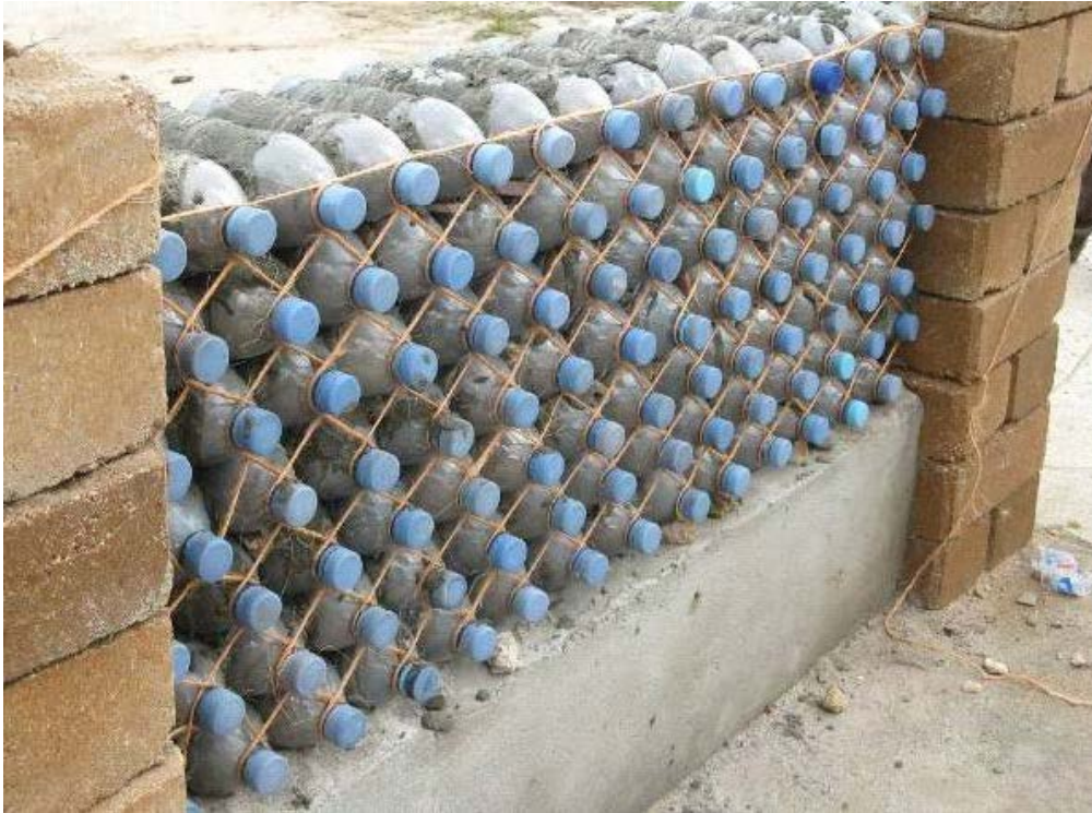
Figure 4.6: The experimental bottle wall constructed in Chamazi. The lower part of it, which was completed one week earlier, was covered with cement plastering. Photo by: Qidi Jiang, 2013
