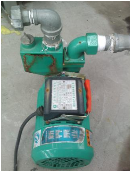
Figure 38: The broken chilling water pump
