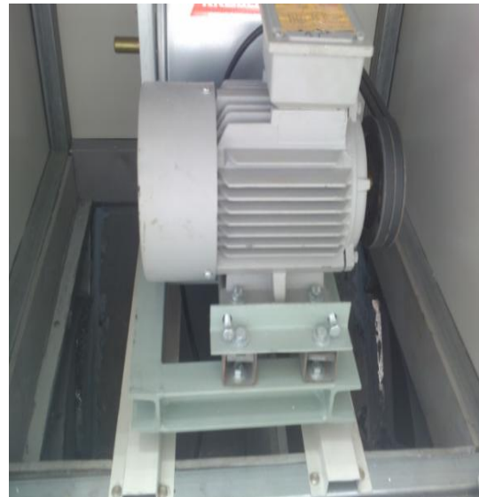
Figure 34: Regeneration air fan
