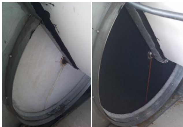
Figure 22: The two desiccant wheels
