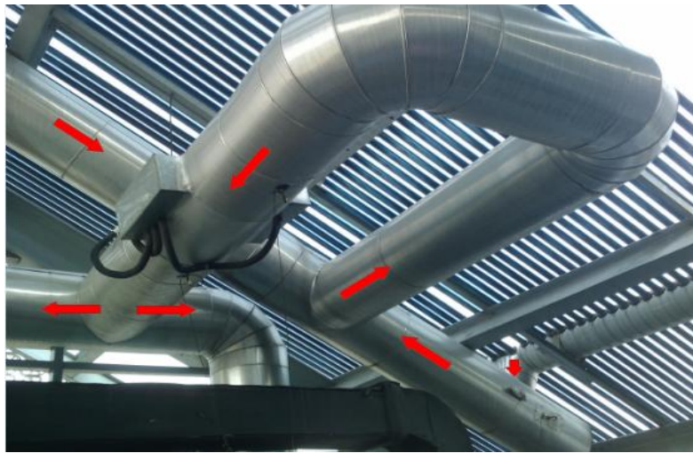
Figure 28: Pipes transferring heated air to the system
