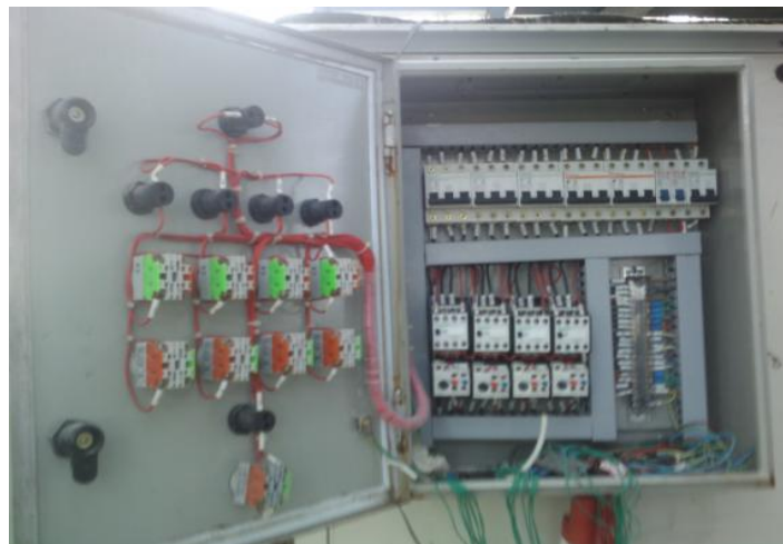
Figure 21: Electrical control locker
