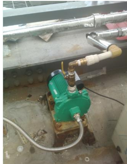
Figure 39: The new chilling water pump
