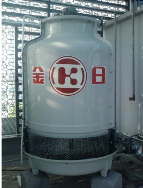
Figure 32: The cooling tower connected to the system
