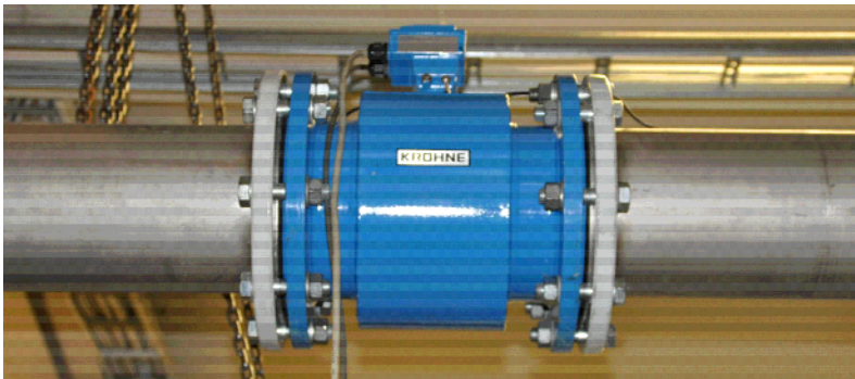
Figure 3-6 The flow meter use in the test
