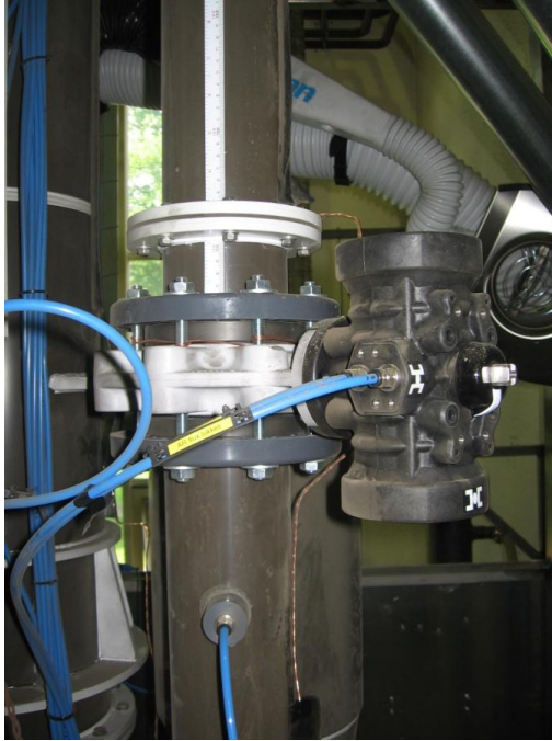
Figure 4-11: Picture of the flap valve which is used in Cold Flow Model rig
