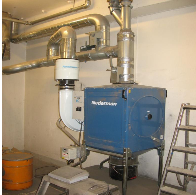
Figure 4-3: On site picture of filter box
