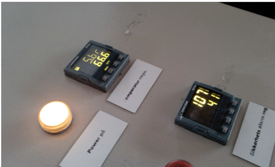
Figur 7-3, Kontrollpanel for effektregulering
