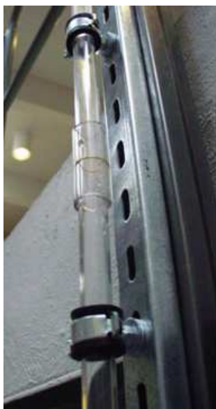
(a) Riser pipes interconnected with flexible hose
