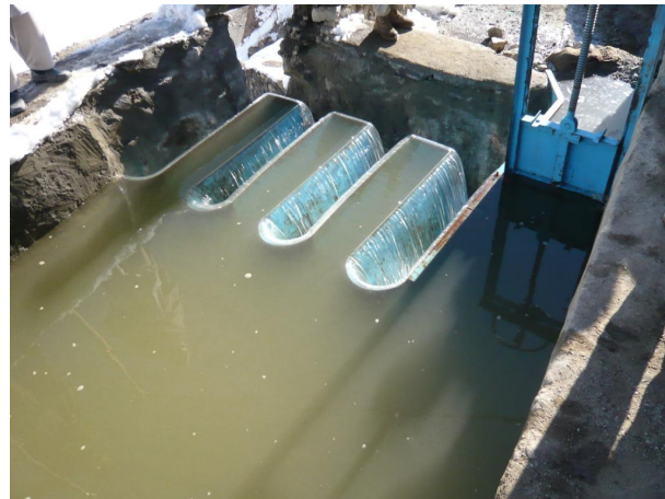
(c) Overflow with gate for applying water to fields
