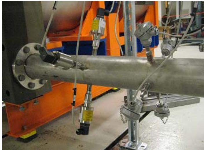
Figure 4.9: Pressure and temperature sensors at outlet
