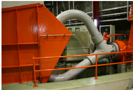
Figure C.3: Inside the machine house in Khimti I.
