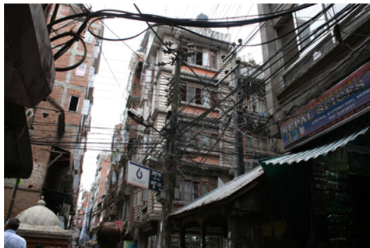
Figure C.4: The electrical grid in Kathmandu.
