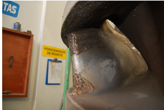
Figure 5.7: The grinded outlet of a Francis runner at Cahua in Peru.
