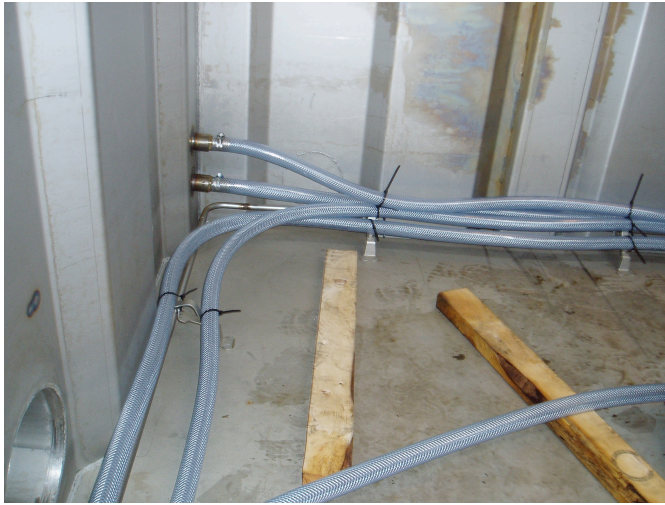
(a) Heating of cargo
