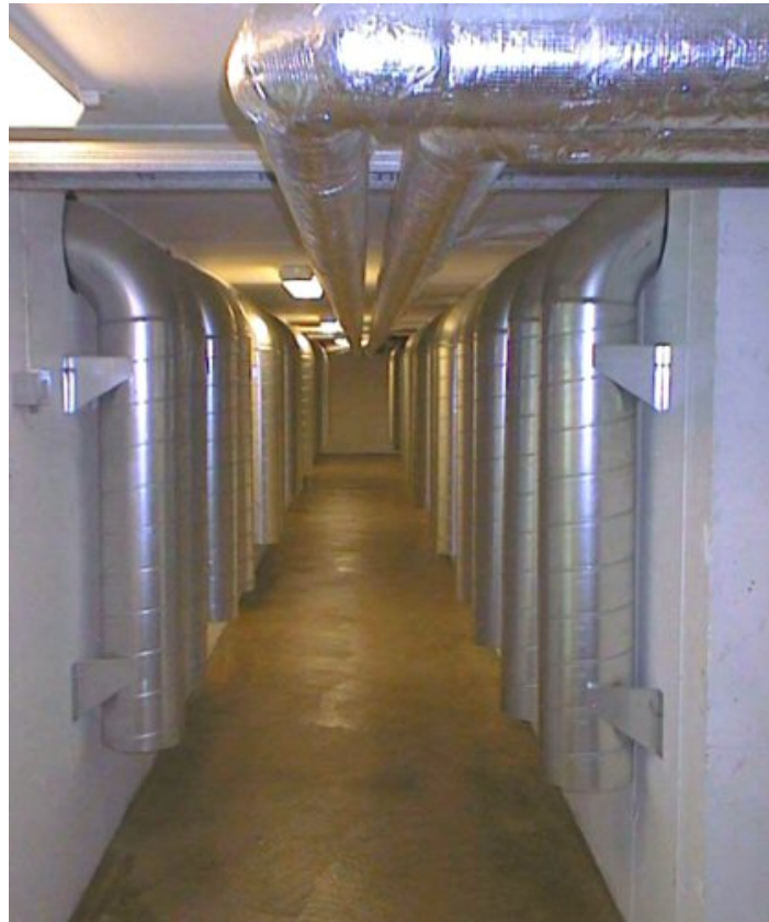
Figure 6-5 Inside of the air distribution culvert, showing the air supply duct stubs. Each duct supplies an office room (Mathisen, 2004)
