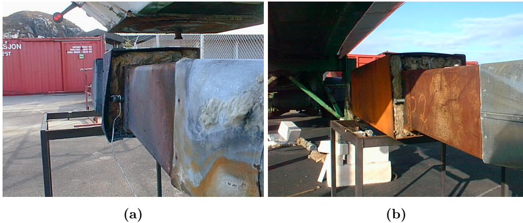
Figure 5.11: Physical condition of extension pipe and insulation material inside encasing on right side of channel (a) and on left side of channel (b)
