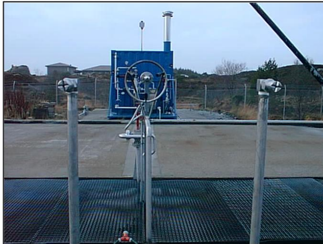
Figure 4.22: Nozzle with 65° spray angle in position, jet fire nozzle in background
