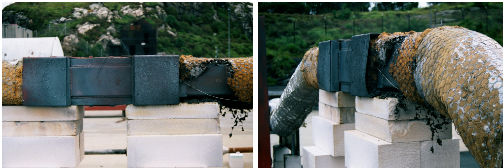
Figure 5.12: Physical condition of external insulation material on right side of channel
