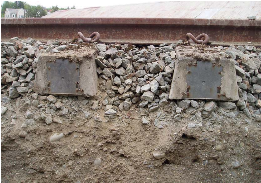
Figure 1.3. Fouled ballast on Stavne-Leangen Line near Trondheim.
