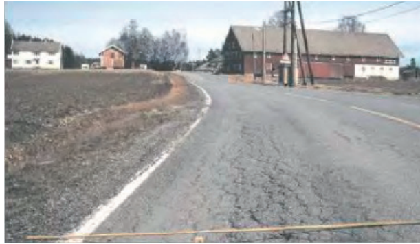
Figure 2.6: Surface rutting with high degree of severity [81].
