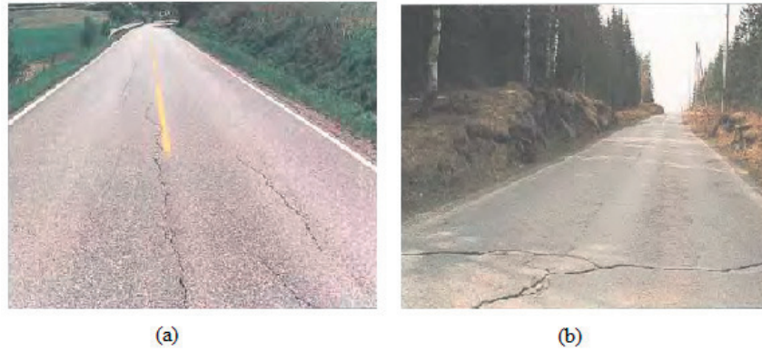
Figure 2.7: a) Longitudinal cracking with medium degree of severity, and b) transverse cracking with high degree of severity [81].
