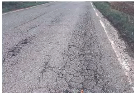
Figure 2.8: Fatigue cracking with high degree of severity [81].
