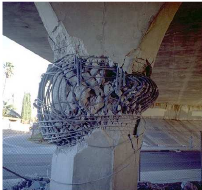
Figure 2.3 Brittleness failure in column.
