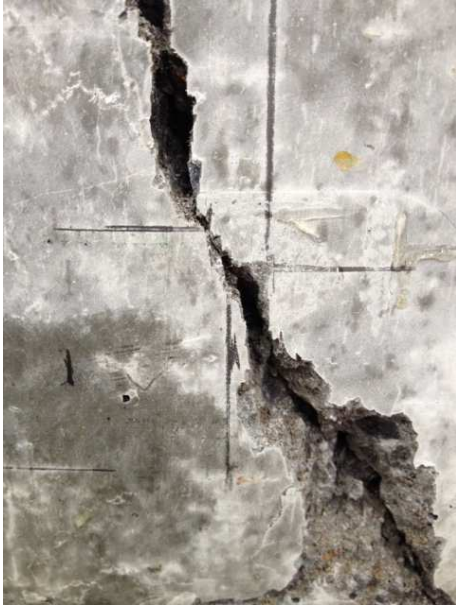
Figure 4.16 LWAC 0,5% B1 centric, Close up of shear band on North face
