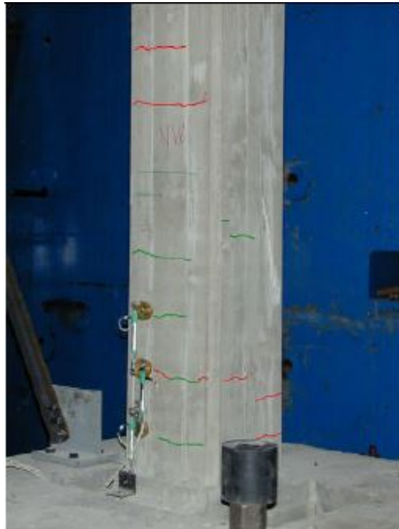
Figure 4.8: Crack patterns on northern frame - western column at the end of 0.64g test (Ferrara & Negro, 2003).
