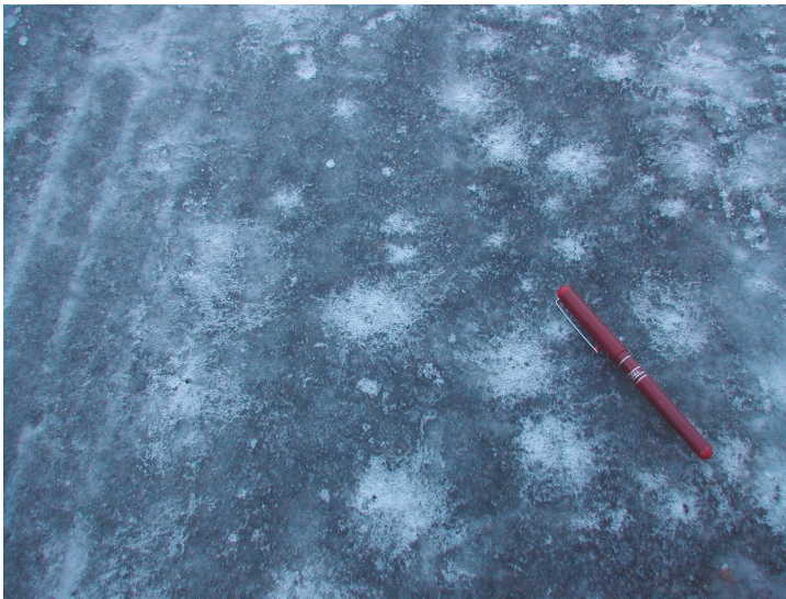
Figure 3.4 Penetration and undercutting on an ice-covered road surface. Photo, Torgeir Vaa (Vaa, 2005).
