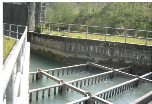
Figure 15 Flow tranquilizers at the inlet of Settling basins in Lower Modi HEP
