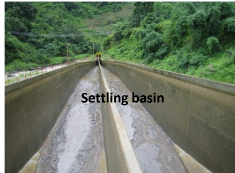
Figure 13 Sediment deposition in the settling basins of Khudi HPP
