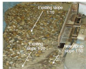
Figure 75 Modifications at the downstream river slope of Khudi HPP (Shrestha et al., 2008)
