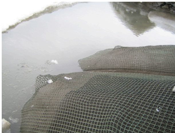
Figure B.106: Deformed protection net at the west corner of the breakwater – 16 June 2007 (week 24)
