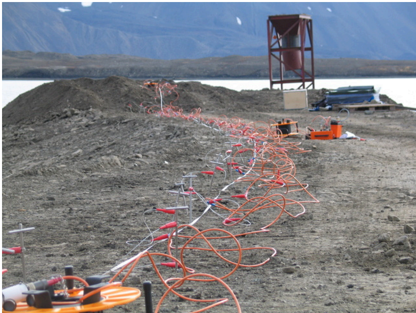
Figure 4.16: Measurement of ground resistivity – 2 September 2006
