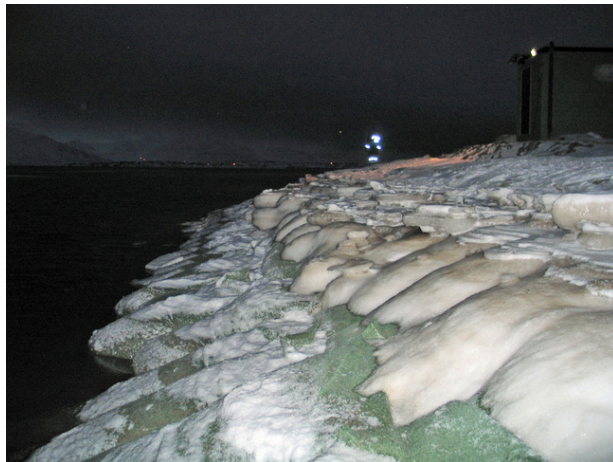
Figure B.14: Bags at the tip of the breakwater, looking toward west, sea height = -0.3 m – 8 November 2006 (week 45)
