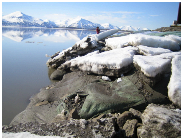
Figure B.113: Damage on bag #150 at the east corner of the breakwater, looking toward west, sea height = -1.0 m – 18 June 2007 (week 25)
