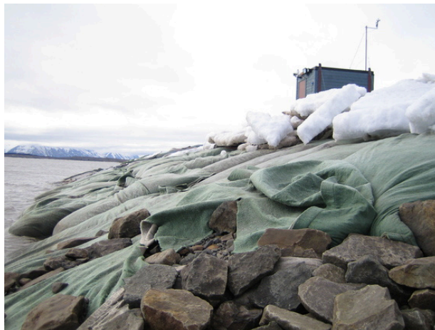
Figure B.119: Breakwater tip, looking toward west, sea height = -0.9 m – 21 June 2007 (week 25)
