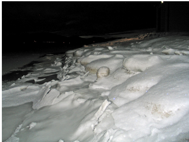
Figure B.19: Bags at the tip of the breakwater, looking toward west, sea height = -0.5 m – 15 November 2006 (week 46)
