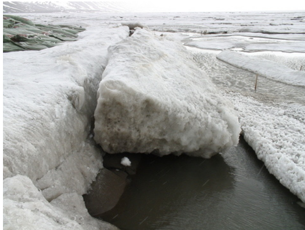
Figure B.95: Ice still attached to the breakwater and crack 1, sea height = -0.9 m – 14 June 2007 (week 24)
