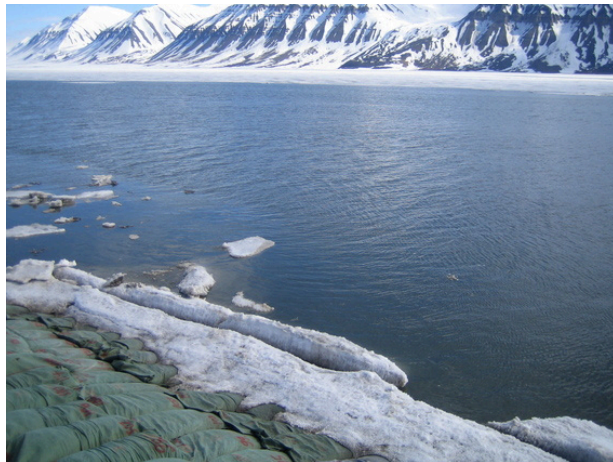
Figure B.98: The area east of the breakwater was ice-free during flow, sea height = -0.3 m – 15 June 2007 14:22 (week 24)
