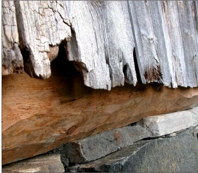
Figure 6.1. Sound ground beam protected with wooden cladding in more than 100 years.
