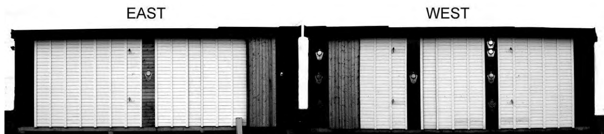
Figure 1.1. The east and west facing facades of the test house, 14 test sections are presented on each side, with varied cavity opening design, growth quality and surface treatment.
