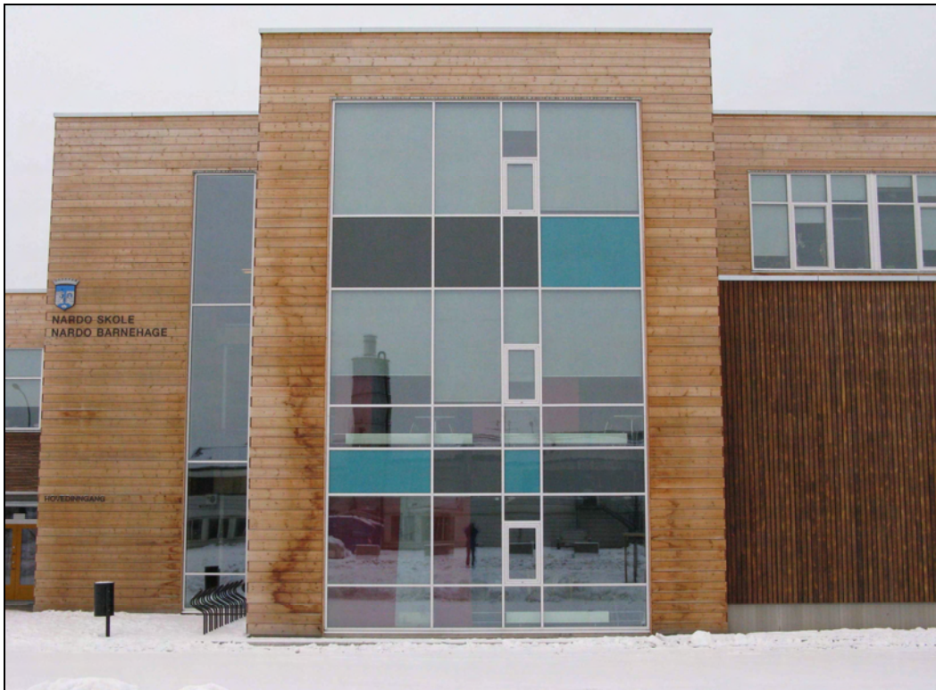
Figure 2.18. Nardo primary school, opened autumn 2008. The cladding has been exposed for one year. Notice the discolourization to the left of the large window. (Photo: Egil Rognvik)
