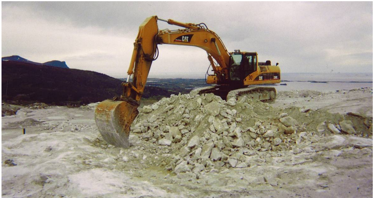
Figure 5 Bench cleaning operation at Visnes Limestone Quarry, Norway. The rock debris from the overlying blast is removed before drilling. Photo: Vegard Olsen.
