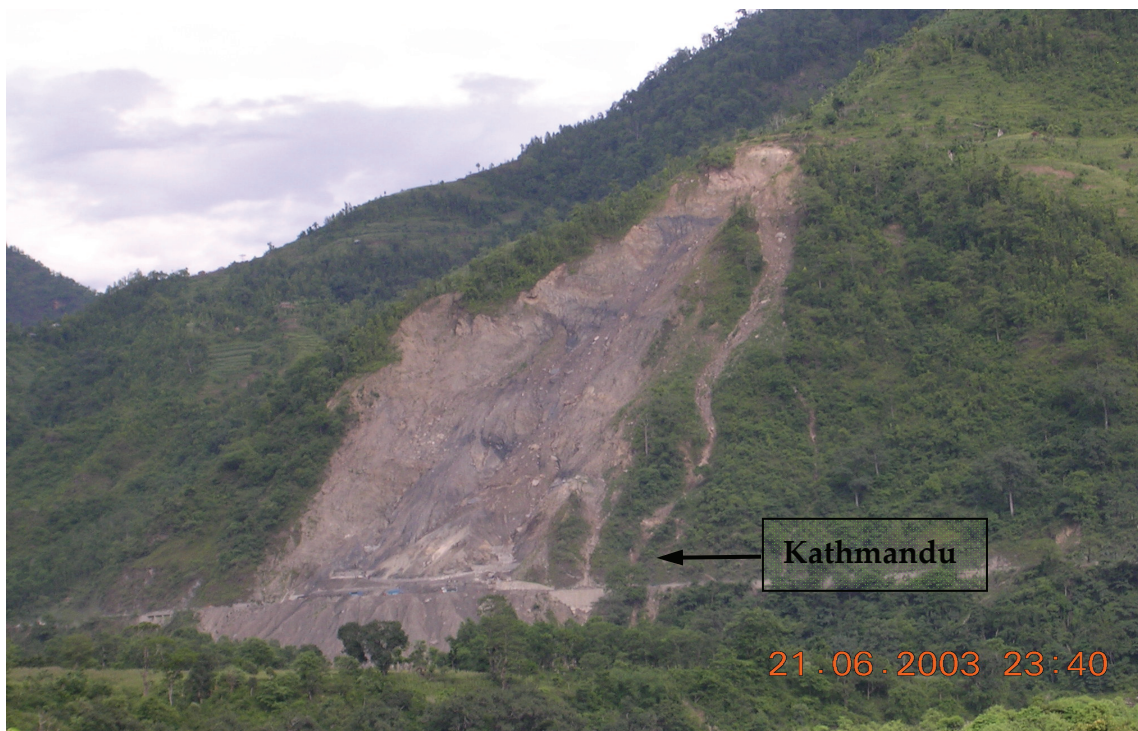
Fig. 1.1 Highway slope failure at Krishnabhir, Tribhuwan highway Nepal (photo from 2003)
