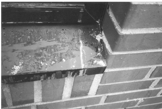
Figure 3c Point of leakage due to the absence of flashing turn-up against a window recess. Source: Norwegian Building Research Institute, Oslo
