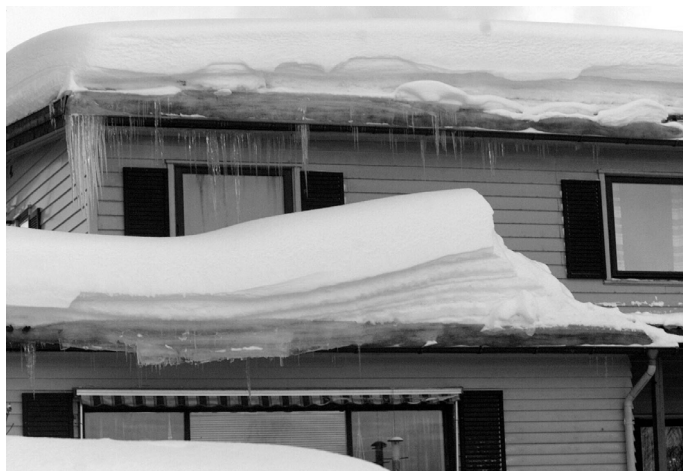
Figure 3. The present design criteria for air gaps have been found to be the risk of ice formation on roofs caused by melting snow (photo: Y.O. Sæbbe, Nordlys).
