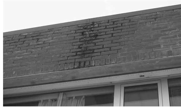
Figure 8 Finishing-off of the parapet flashing against the wall face has led to wetting/moistening of the facade with consequent organic growth. Source: Norwegian Building Research Institute, Oslo
