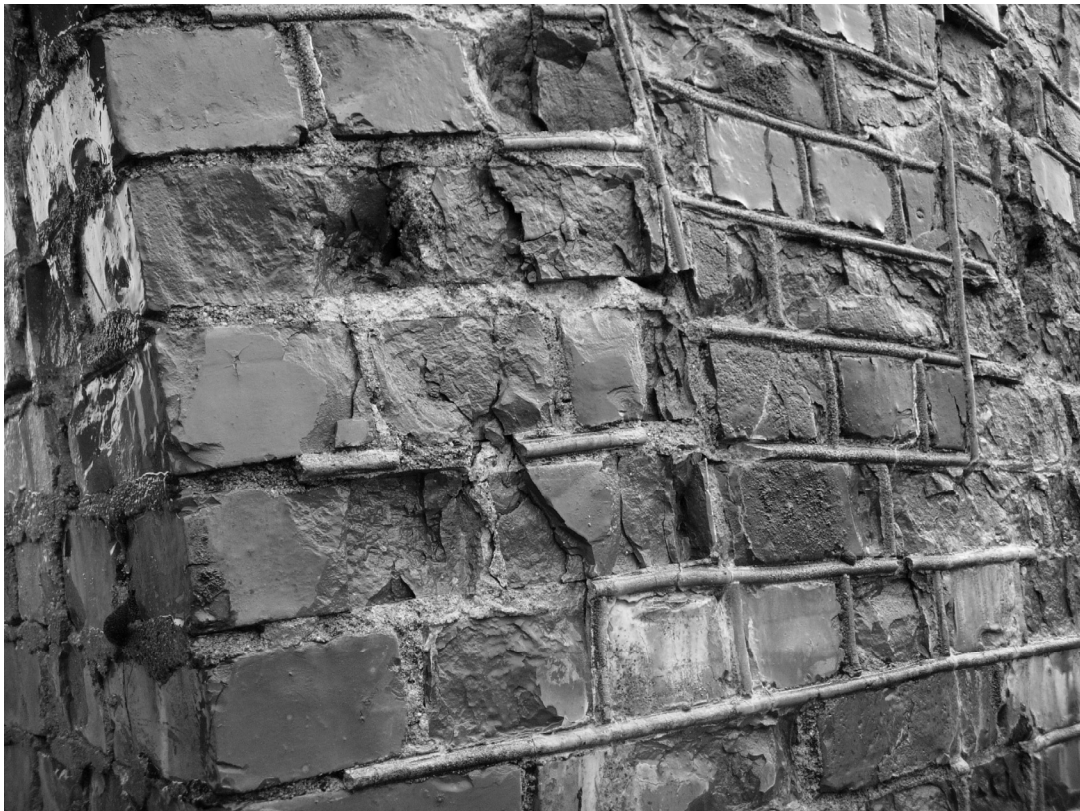
Fig. 3. A frost damaged brick wall (photo: NBI).
