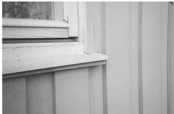
Figure 3e Poor solution where the wood cladding is brought into contact with the windowsill flashing. In addition, the end turn-up is missing. Source: Norwegian Building Research Institute, Oslo
