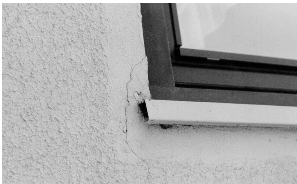
Figure 3a Unsatisfactory rendering around windowsill flashing causing cracks. Source: Norwegian Building Research Institute, Oslo
