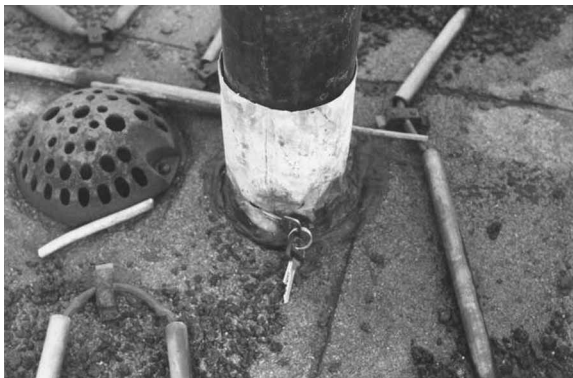
Figure 11c Collars without protective flashing can give rise to severe leakage. A perforation in the flange transition, as in this case, makes the situation even worse. Source: Norwegian Building Research Institute, Oslo
