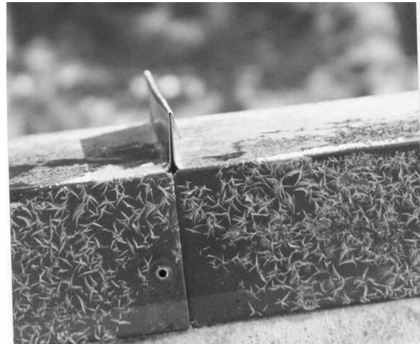
Figure 1 Poorly executed folded welt on parapet flashing. The under-flashing is missing. Source: Norwegian Building Research Institute, Oslo
