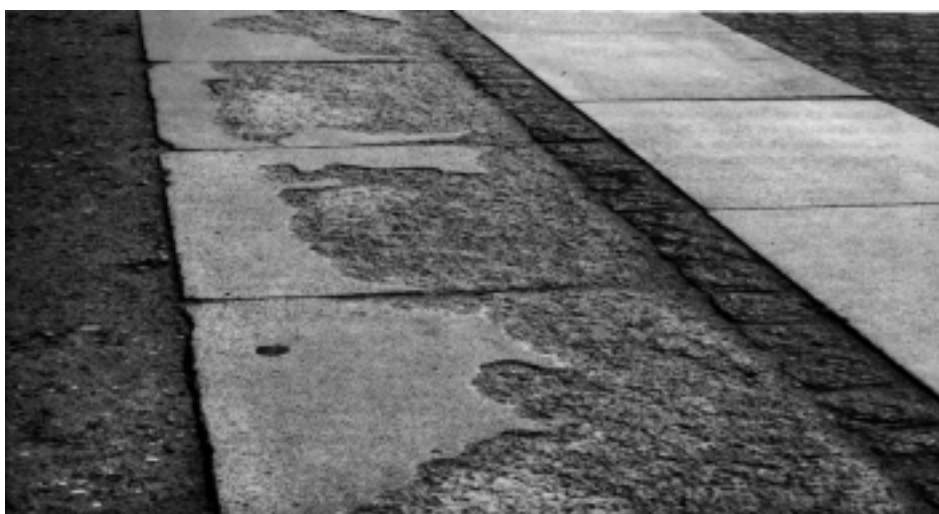
Figure 2.2.1 : Surface damage on a concrete pavement [P 1985].
