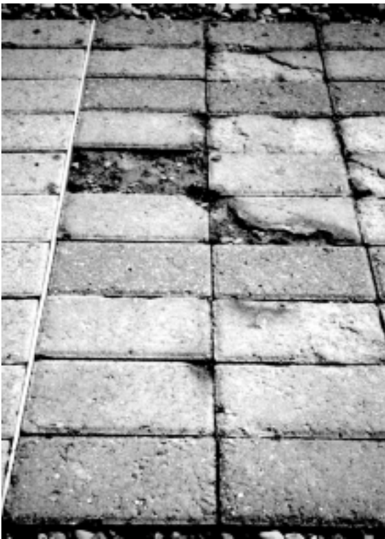
Figure 2.2.6 : Freeze-thaw damages of concrete flags at an outdoor testing facility.
