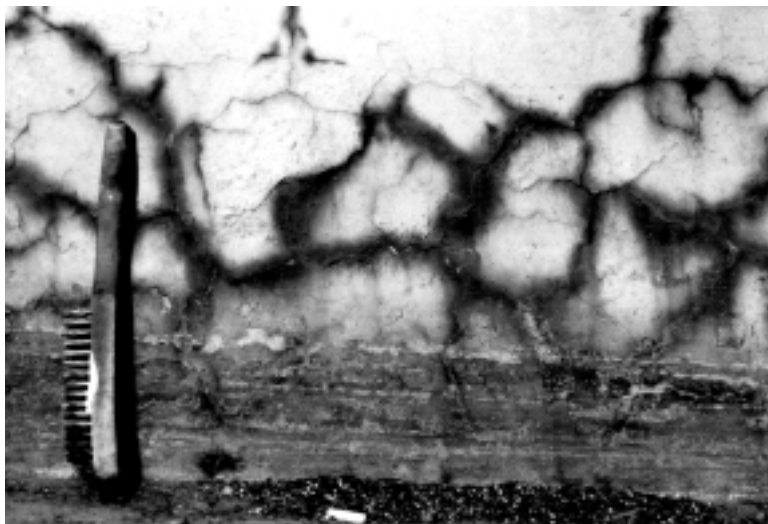
Figure 2.2.7 : Damages at a minor road safety barrier. The damage is not proven to be frost damage, but exhibits 10 cm deep cracks without alkali-aggregate reaction being identified.
