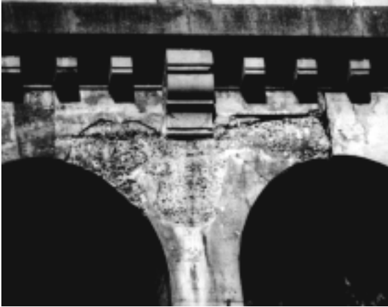
Figure 2.2.5 : Frost damage on the side of a bridge, near Washington D.C.
