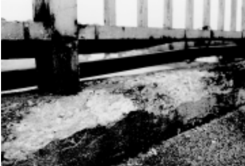
Figure 2.2.3 : Concrete damage at a vulnerable part of a bridge section, exposing the reinforcement to corrosion conditions. Near Vordingborg, Denmark.
