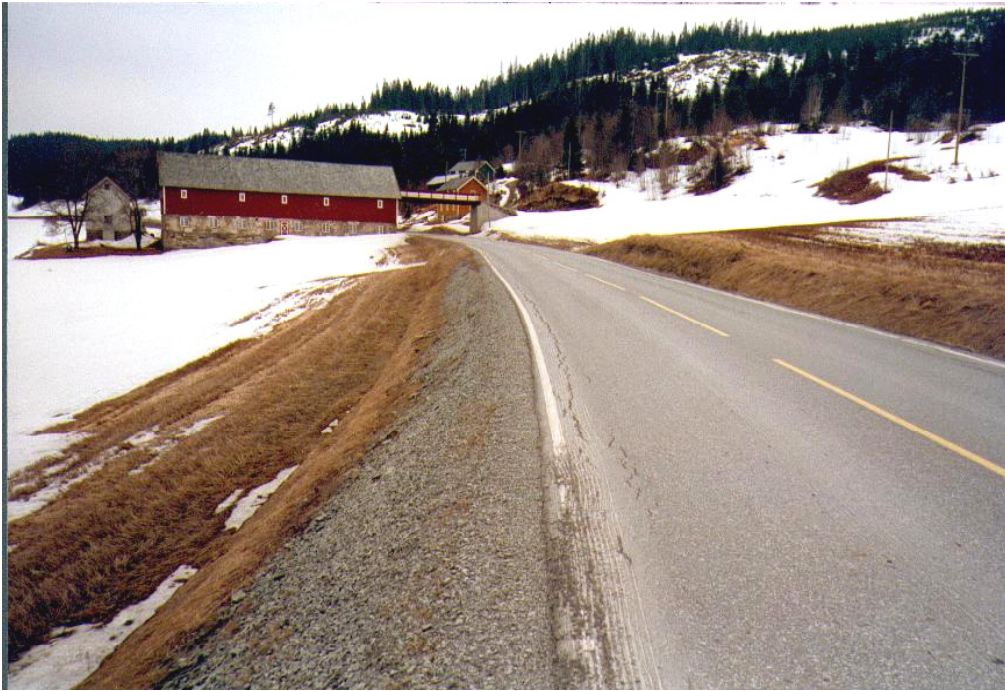
Figure 3-3: Longitudinal cracking along the pavement edge
