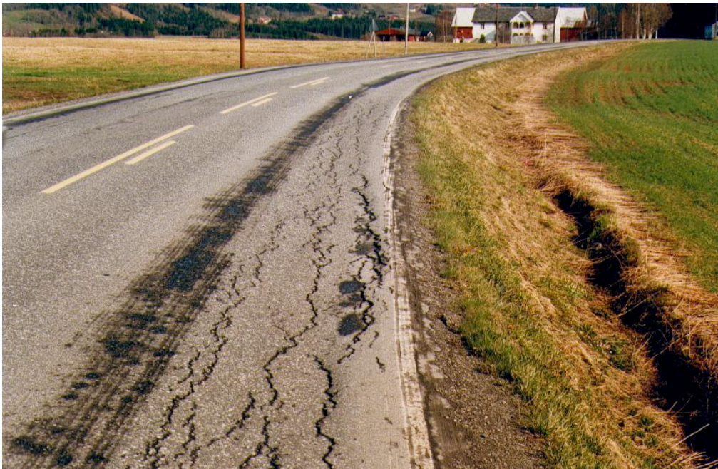
Figure 3-6: Deformation and interconnected longitudinal cracking
