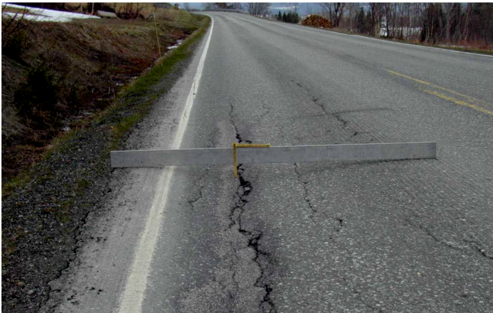
Figure 3-4: Deformation and longitudinal cracking
