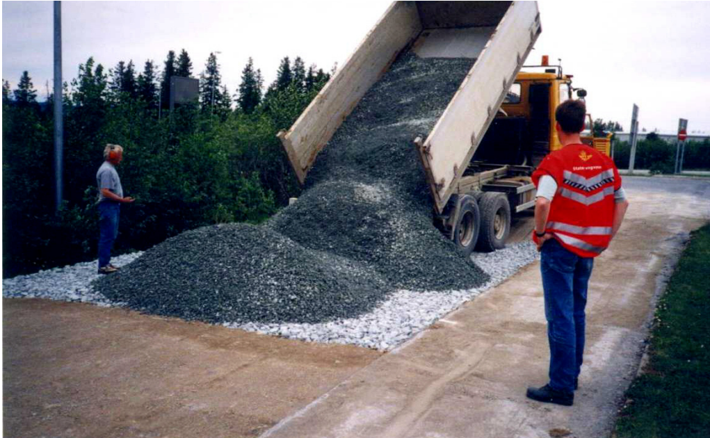
Figure 4-7: Tipping of base material at Section 1 (in the lower left corner of the picture the surface of the subbase layer of Section 2 can be seen)
