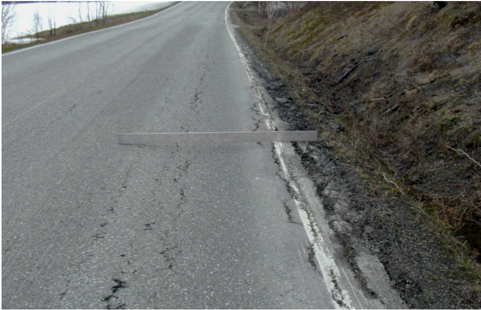
Figure 3-1: Example of severe deformation of outer wheel path
