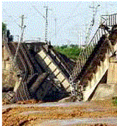
(d). Bridge is broken by flooding
