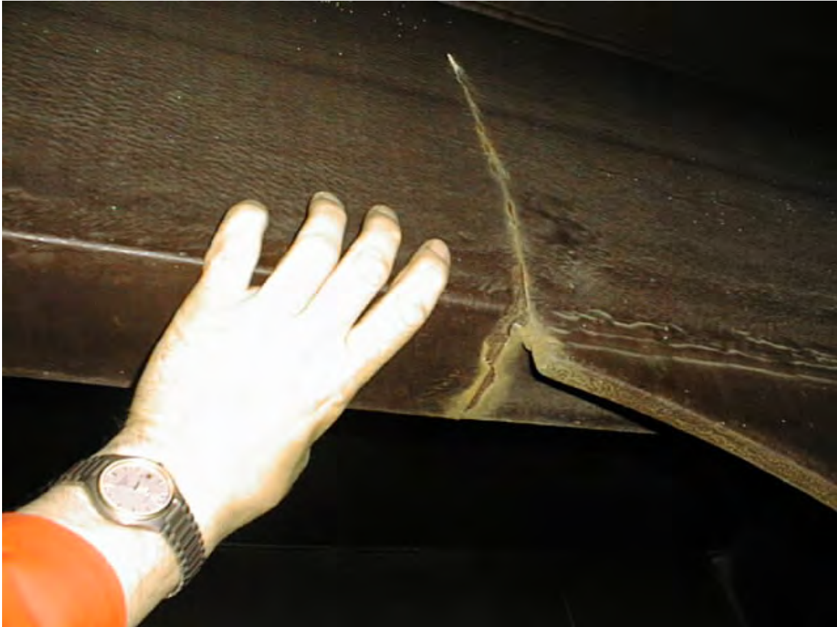
Figure 1.2: Picture of a longitudinal stiffener in deck in way of the transverse bulkhead, and located in the ballast tank. The crack originated from the bracket toe termination.
