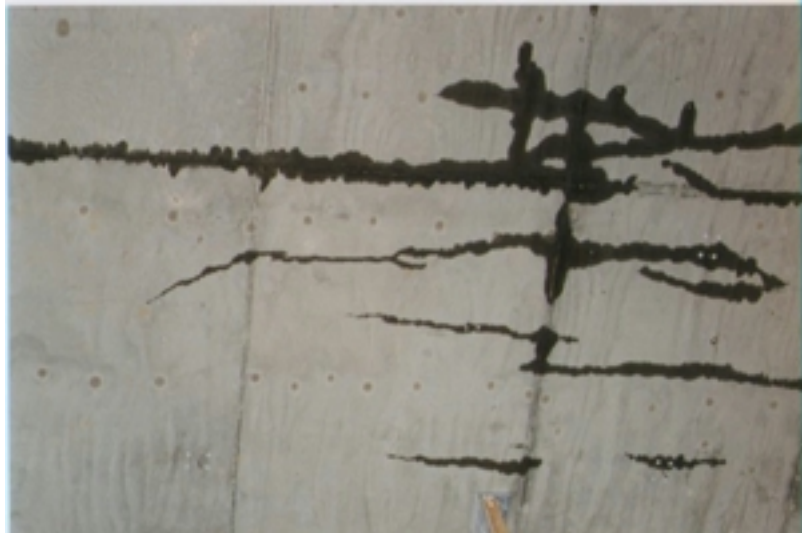
Crack in the bottom of the slab after failure.
