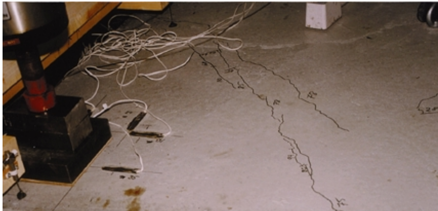
Crack pattern with load in the corner, S3.
