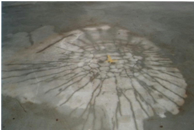
Crack in the top of the slab over the middle column.
