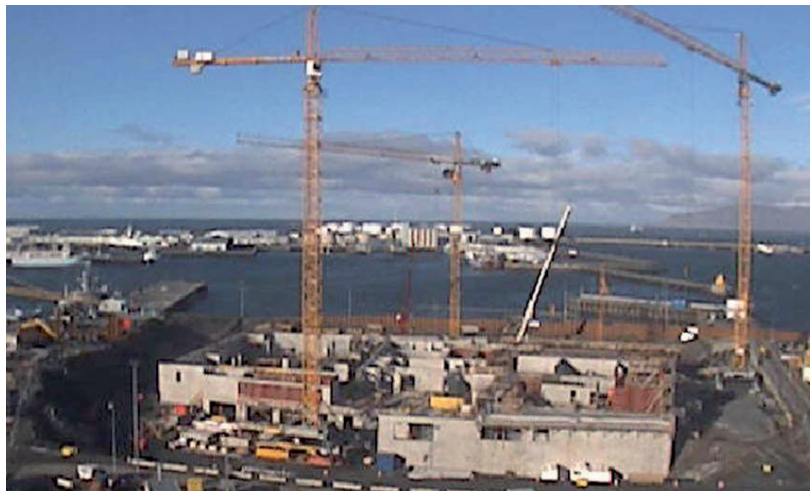
Figure 6-18. Web-cam from the construction site in Reykjavik East Harbor (retrieved October 15th 2007 from the Portus-webpage: http://www.portusgroup.is/video1.html ).
