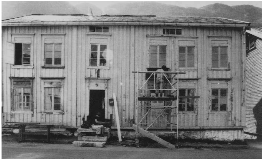
Figure 60: Sjøgata 37, street façade during regeneration. (Photograph Dag Nilsen, Dag Nilsen private archive)
