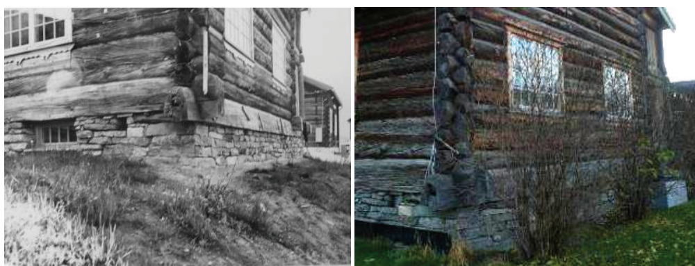
Figure 29-30: Stensgård relocated on new foundations, concrete underground and natural stone above, in 1978-80 (left) and in 2008. (Photograph unknown©Riksantikvaren and MB 2008)
