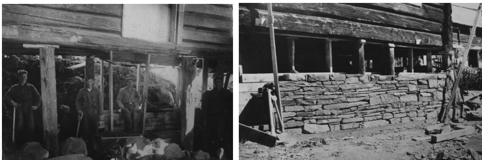
Figure 50-51: Søndre Stugu. "Ungdomsopplæring i arbeid" ("Youth training at work") State employment grants used to repair listed buildings. Work on the foundations of Søndre Stugu at Harildstad Søre in 1938 were prescribed and inspected by Halvor Vreim. (Photographs Halvor Vreim ©Riksantikvaren)
