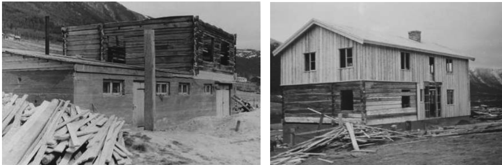
Figure 11-12: Krogstad under construction in 1956 showing the new cast concrete basement (left) with the garage doors and the notched case with the three rooms; and from the opposite angle (right) with the new addition and visible signs that the old construction was repaired with new sills and back wall logs fitted. (Photographs: Halvor Vreim ©Riksantikvaren)
