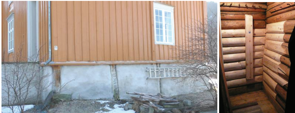
Figure 14-15: The west end, exterior (left) and section of wall in the upstairs clothes chamber (right) viewed from the interior (right). In 1758, only 14 years after the west end (with Borgestuen and Størhuset ) was built, its foundations were considered so unsound that taking apart and reassembling this whole section was considered. In 1814 it was noted that the outer stairs (far left in left-hand photo) were timbered; today they are stone. 113 By the stairs to Størhuset a hole in the wall was observed in 1802, which would require “planks and nails”. 114 This hole was still there in 2000, when it was discovered that the entire log wall section had been subject to a serious fungal attack. In the clothes chamber (right) a fossilized fungus was found, likely produced by the leakage which was described in 1802. About 50% of the wall timber was renewed after the year 2000. (Photographs MB 2007)
