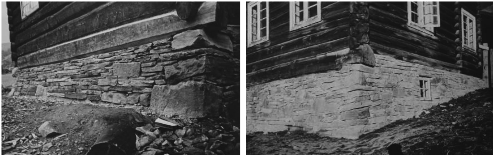
Figure 52-53: Nordre Stugu “The new foundations under the northern dwelling” (left) and Nedre Stugu (right) photographed by Vreim in 1939. On both buildings the foundations were repaired. The photo of Nordre Stugu was presented in the piece Fortidsvern og ungdomsarbeid in Fortidsminneforeningen ’s 1939 annal with the caption “House lifted and provided with new foundations and bottom logs. The old stone re-used, but with reinforcements at the back.” 208 (Riksantikvaren archive)
