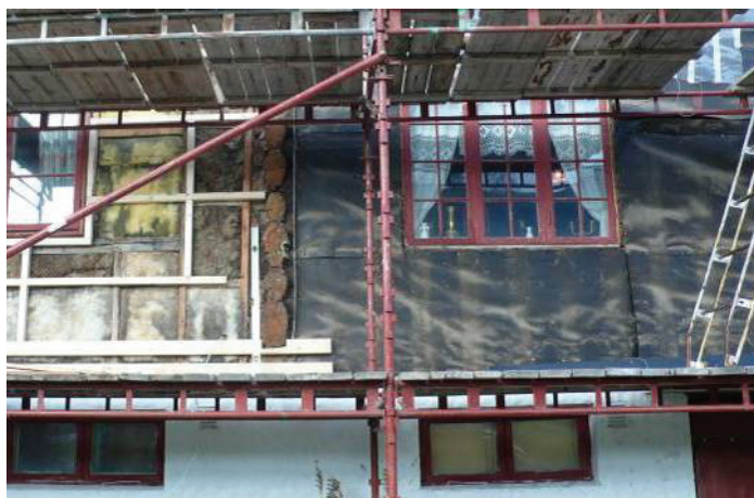
Figure 9: Krogstad søre, 2008. The boarding removed, exposing 1950s type wind-proofing on the 1811-section of the building. Vreim had strongly recommended that this section was to be left with exposed timber. Initially this was the case, but apparently not for long. (Photograph MB 2008)
