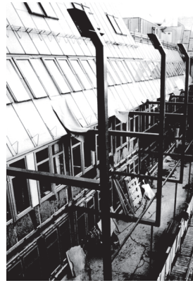
Construction works, extension to 4. - 6. floor. The façade could not support the extra weight, so a system of internal pillars was constructed (photograph by Jens Barland).
