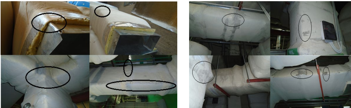
Figure1: Compression of duct insulation (left) and accumulation of water vapor at the point of compression (right).
