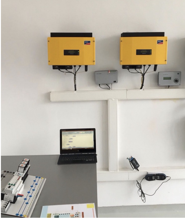
FIG. 3: Inverters and WebBox equipment for the monitoring and data acquisition of the PV system
