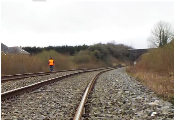
Figure 5. Track settlement location. (Photograph: C. Bowe).
