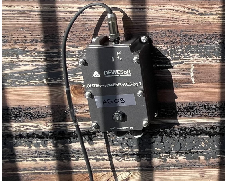
Figure 8: One of the accelerometers installed on the bridge.
