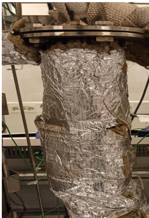
Figure 35: Hot gas filter with insulation.
