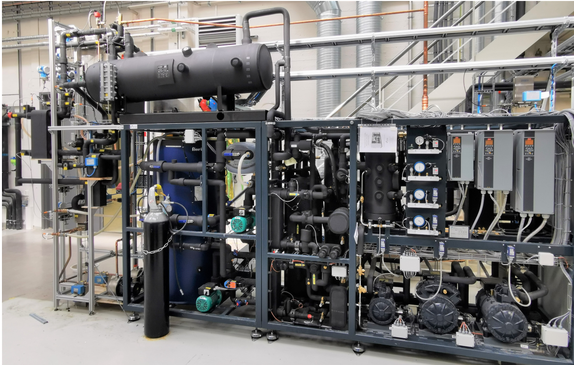
Figure 13: The Multifunctional test-rack
