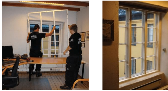
Figure 3.1: Installation of a secondary glazing improving the window's U-value from 4.6 W/(m 2 K) to 1.6 W/(m 2 K). Photo: Marte Boro (Directorate for Cultural Heritage, n.d.).
