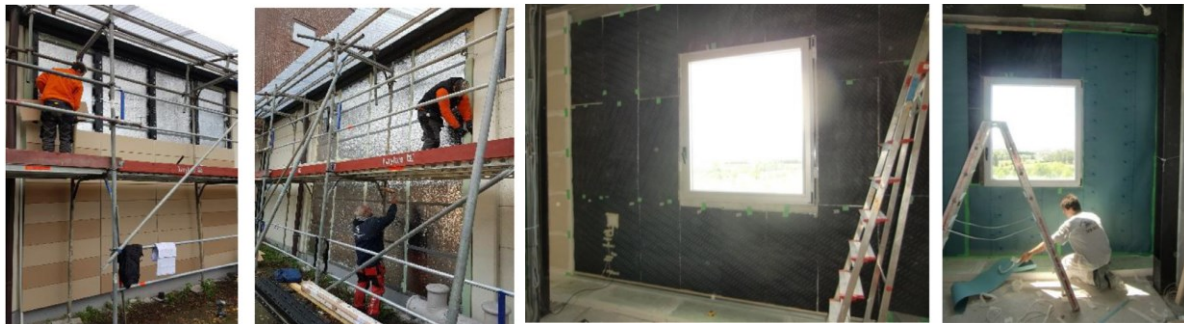
Figure 4.2: External ventilated façade retrofitting with VIPs in Malmö (two left photos) and internal installation of VIPs in KUBIK by Tecnalia (two right photos) (Uriarte et al., 2019).
