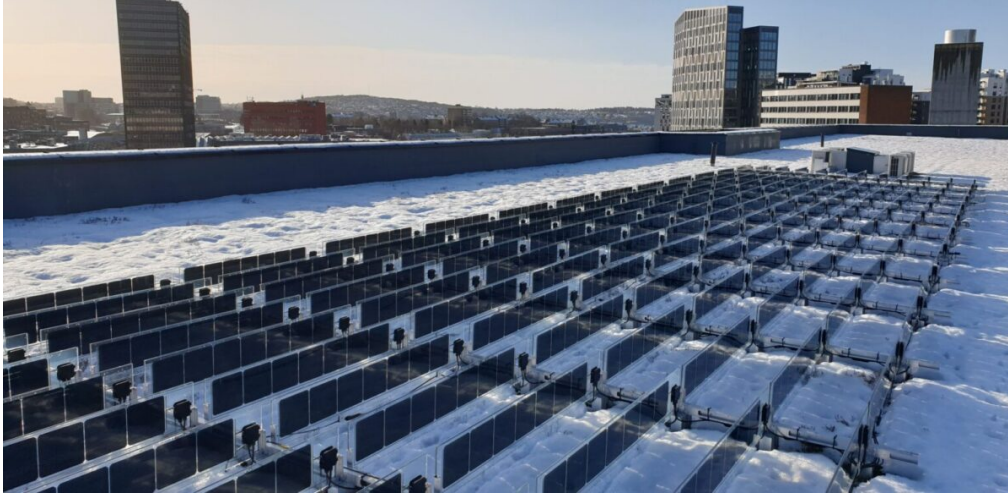
Figure 3: Over Easy Solar vertical bifacial pilot installation in Oslo, Norway [19].
