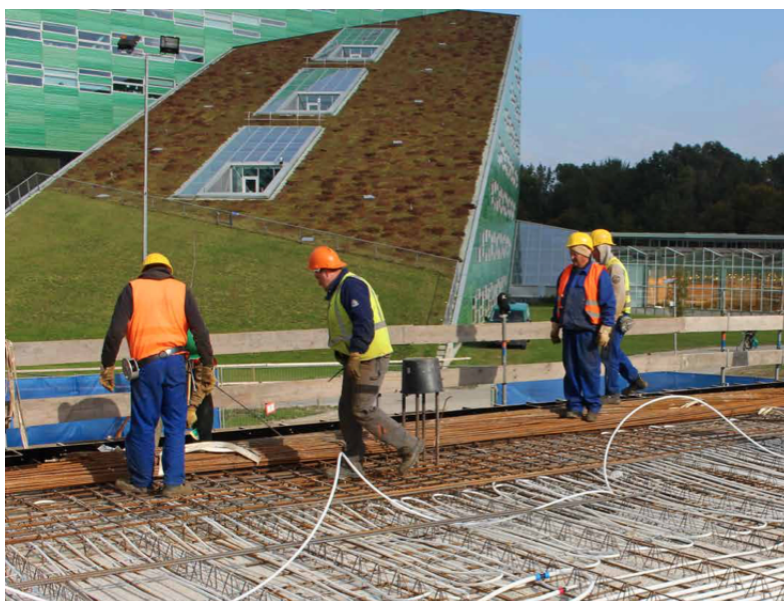
Figure 4.2.12: Under-floor heating and cooling system ( Energy Academy Europe , 2017)
