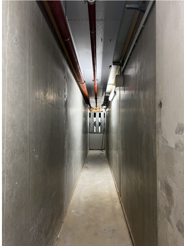
Figure 4.2.9: The walls of the labyrinth heat or cool the ventilation air, Photo taken by the author.
