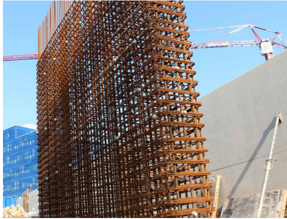
Figure 4.2.15: Six seismic walls are in place to absorb possible earthquakes ( Energy Academy Europe , 2017).
